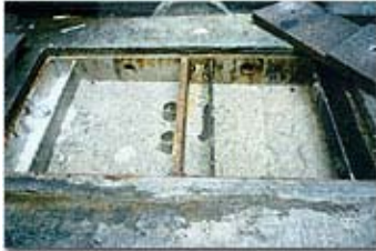
An Underground Grease Trap of a Restaurant
